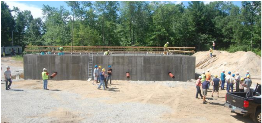
Above: Merrimack Village Water District's new 1.8 MGD iron and manganese removal treatment facility.
