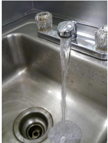
Figure 2: Public Sampling Point with Aerator Removed
