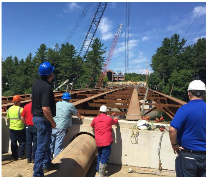
Above: After lunch at White Park in Concord, the bus traveled to Penacook to visit a water main replacement project and then on to the Sewalls Falls Bridge project.
