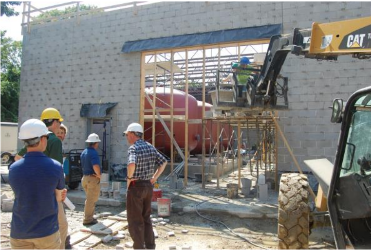
The Lowell Avenue water treatment plant going up around the new filter tanks.
