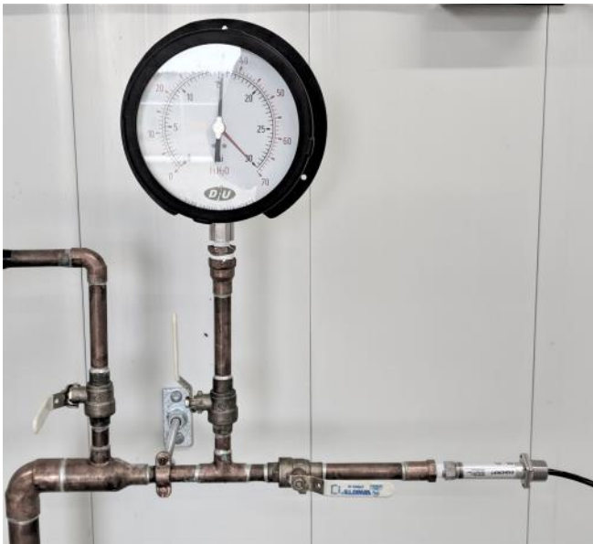
Tank level gauge and tank level transmitter
