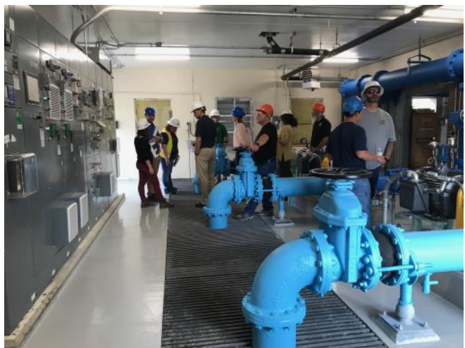
Inside the Newington Booster Pump Station.
