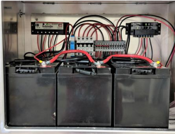
Solar panel controls and batteries
