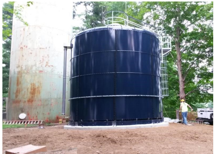
The Newfields Water Department recently completed the construction of a new .25MG Aquastore storage tank.
