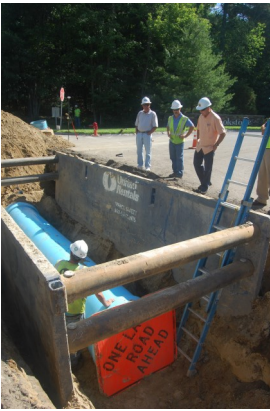
Pennichuck Water Works' transmission connector.
