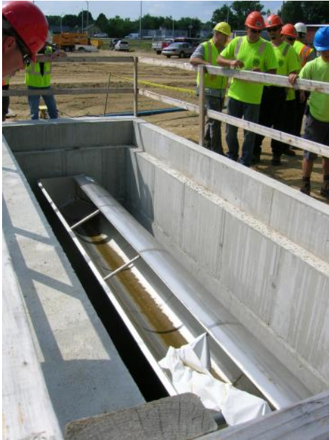
Nashua's combined sewer overflow project "Drain Chamber".
