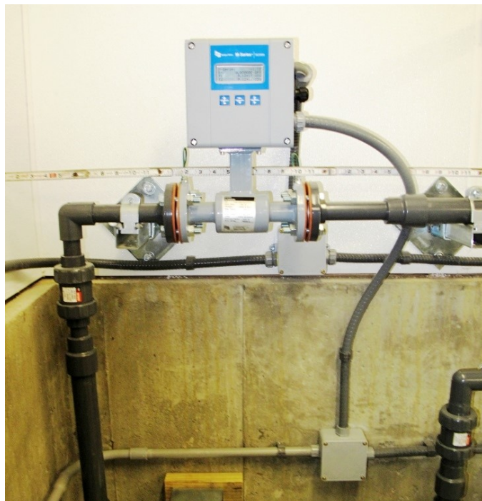
Well 1 entrance at Mittersill Water System.
