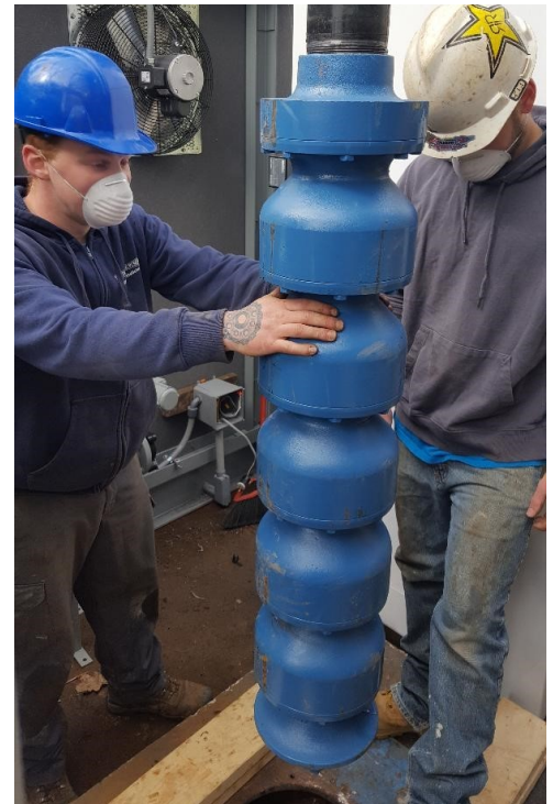
Epping Well and Pump technicians wear personal protective equipment while installing a turbine pump.
