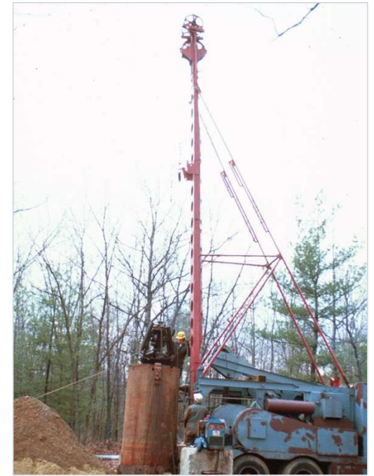
48 inch, only 10% increase In Yield w/Doubling Well Diameter
