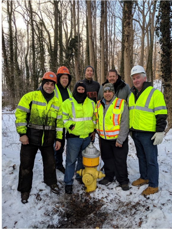
iHYDRANT™ | INSTALLATION, NY
