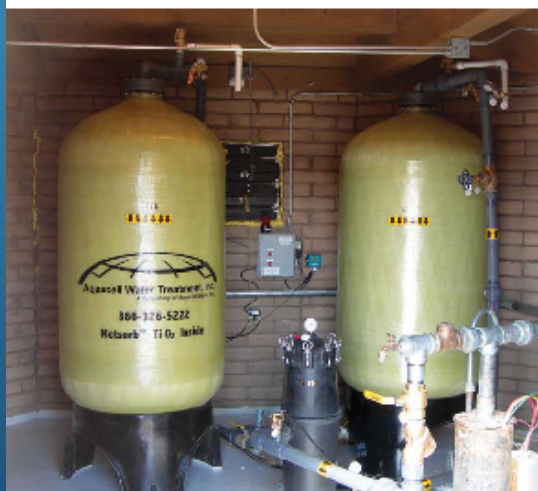
Dual vessels containing MetSorb plumbed in series for added consumer protection
